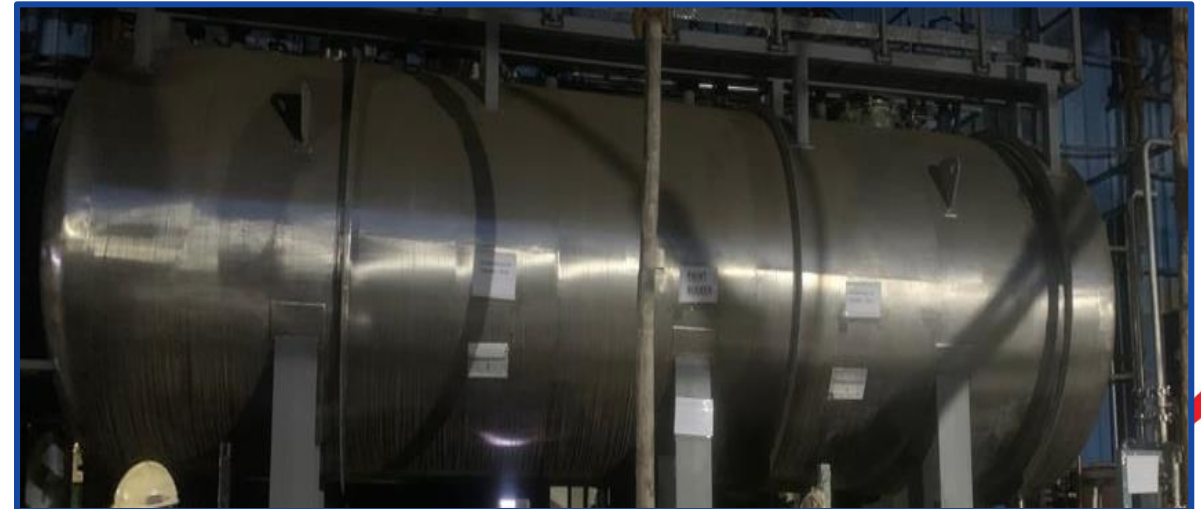
Use of Paint Bulker at Color Coating Line
